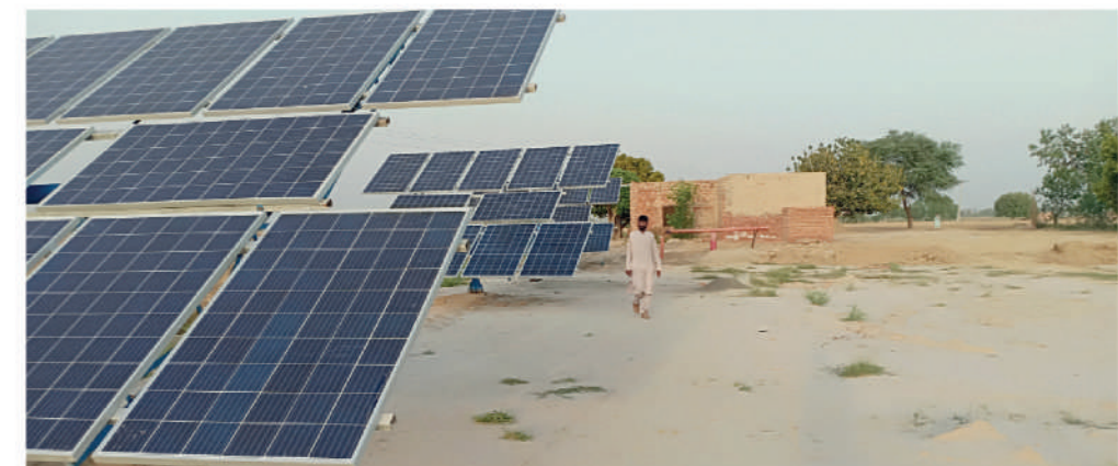
Solar panels installed as part of KMP ensure reliable and affordable alternate source of energy for the farmers.
