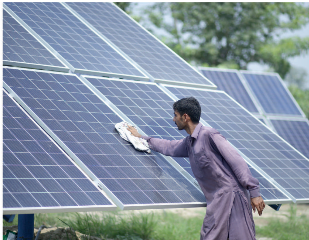
COs pooled resources and took interest-free loans to install solar panels which power shared tube-wells
